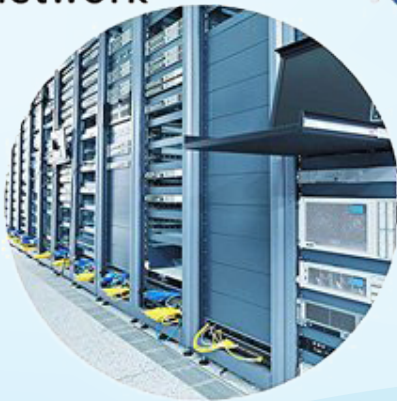
Network control room
