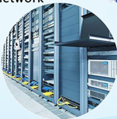
Network control room
